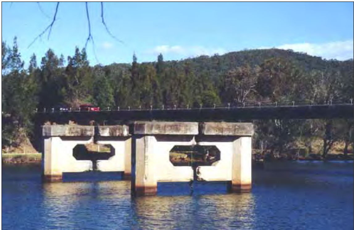
Plate 11: Site H21 - pylon remains of former concrete Pacific Highway bridge – looking south from N bank of Camden Haven River.
